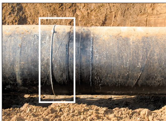
Fig. 9. Widening of a pipe after the stress test
