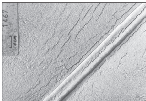
Fig. 6. Stress corrosion cracking on the inner pipe surface [8]
